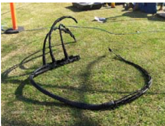
Crews pulled melted wire, conduit from exterior vault.
