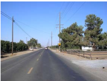
Radar vehicle speed feedback signs we installed east and west of Hope Elementary School.
